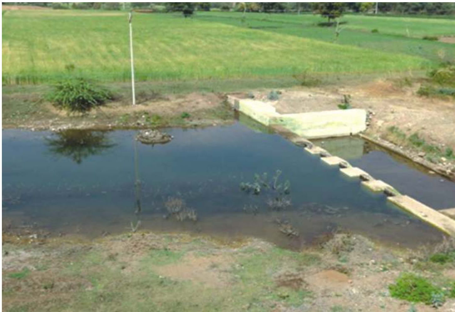
Masonry Stop dam constructed 10 years ago irrigating the Rabi crop in Jhabua district, Madhya Pradesh.
